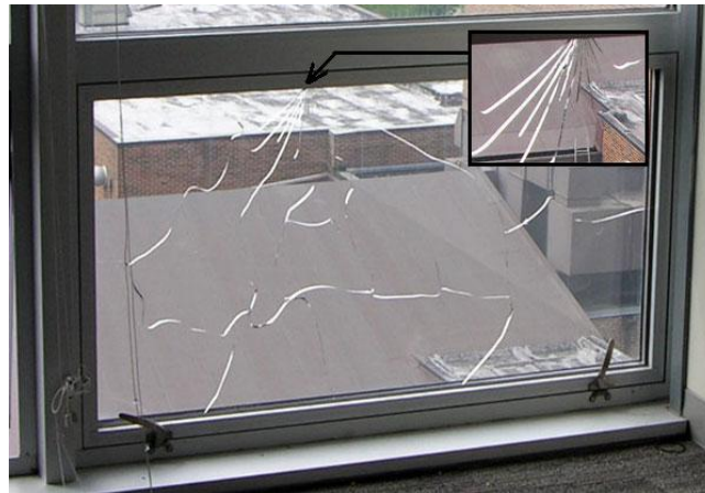
Photo of broken glass. Classic meandering pattern of heat-related stress crack accompanied by evidence of edge damage. In this case, the glass had both: edge damage and underspecified glass. In addition, reflective blinds and a South exposure combined to create a high frequency of this type of breakage.
