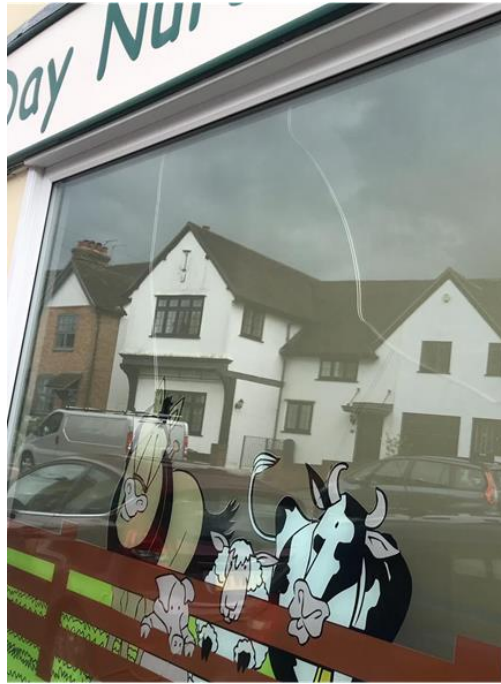
Photo of two cracks present in the outside face of a double-glazed unit. Vinyl graphics applied to the lower part of a window.
